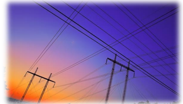
35kV over head transmission line
