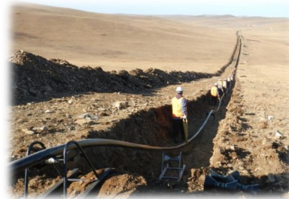
35kV underground cable network of Salkhit wind farm
